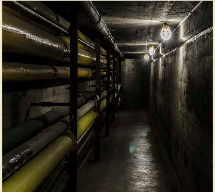
Aged steam pipes at Victoria Hospital
